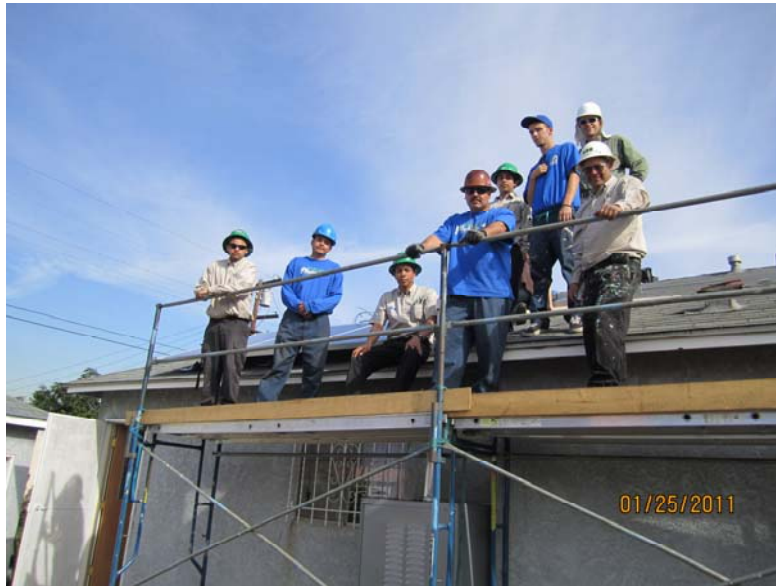
Shows LACCN Corpsmembers, Supervisors and installers from Grid Alternatives at the installation in Compton.
