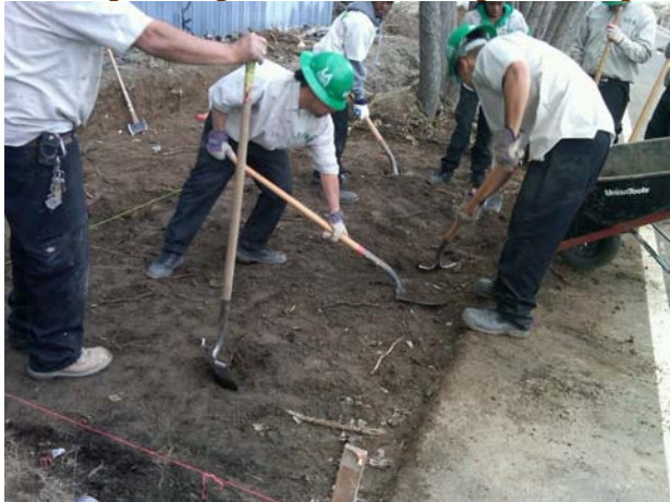
Andy Diaz, Jeffrey Scott, Alicia Johnson, and David Sanchez preparing for installation of equipment
