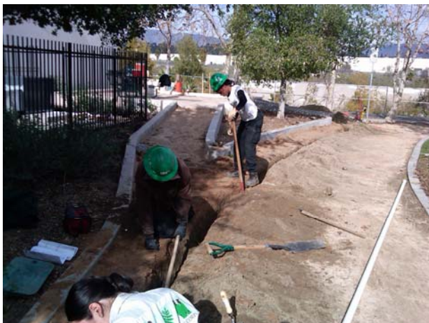
Gardenia Romero, Jaime Llamas, and Alicia Johnson installing the main line pipe
