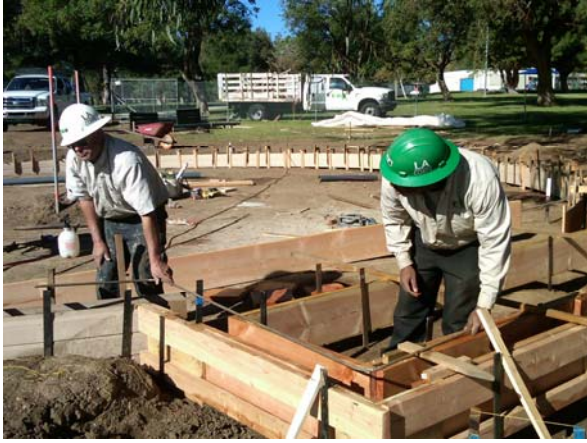
Corpsmember Dean Payne working with Frank on a technical section of concrete forms
