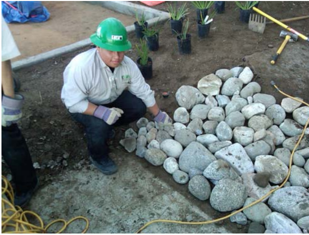
Corpsmembers used river rocks to create a rip rap for storm water run off
