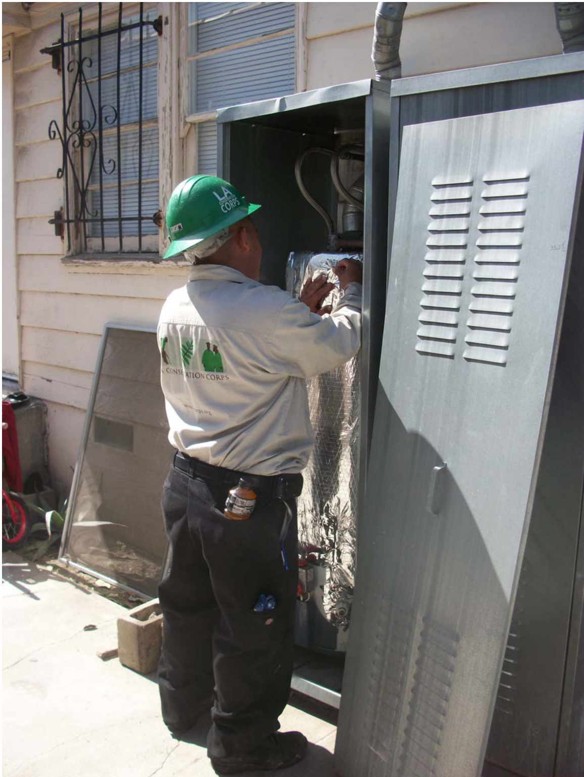
Solar crews completed their fourth installation for Grid Alternatives last week. The installation was scheduled for two days but our crews only took one (photo below). Good job!
